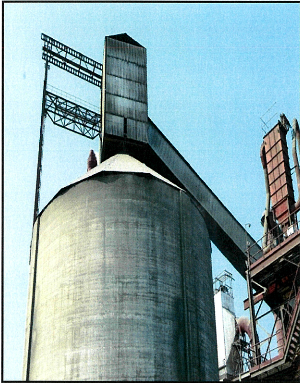
Line 3 Clinker Silo
