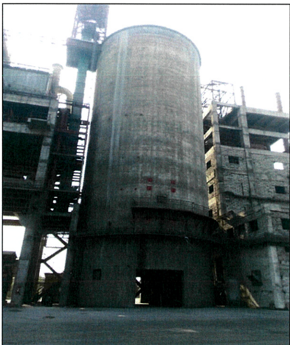
LINE 3 Cement Silo
