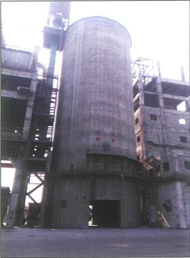
LINE 3 Cement Silo
