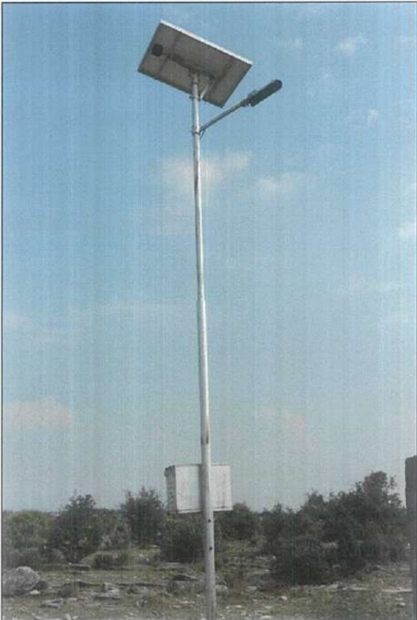
SOLAR PANEL LIGHTING SYSTEM
